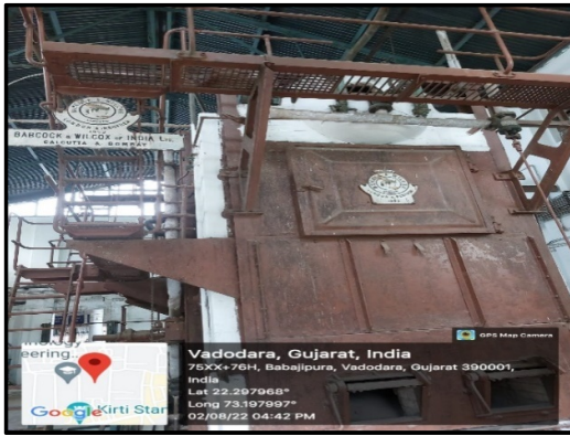
Babcock Wilcox Boiler
